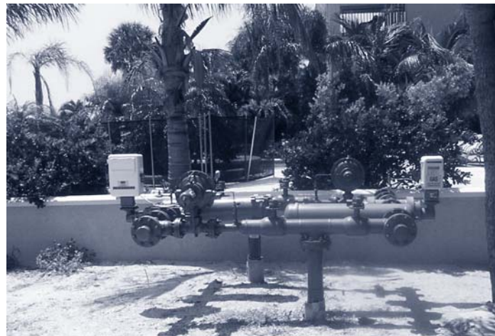
The CGS Redington Beach interconnect facility supports service to natural gas customers during low pressure situations.
